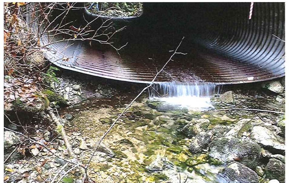
CK2334 Left Pipe Outlet
